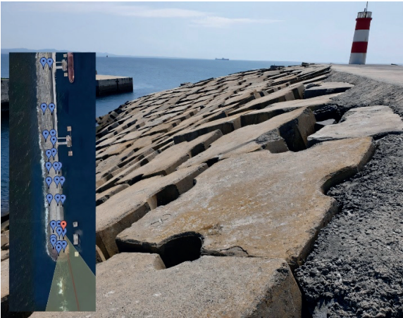
Figure 7. 2020 visual observation at point 28F of the Sines west breakwater (inner armour layer)
