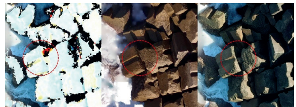
Figure 19. West breakwater. Changes detected between 2020 and 2022 – Occurrence 2 – Section E
