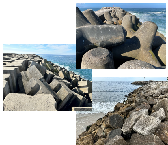
Figure 1. Breakwater armour layers composed of: (a, b) concrete units (Ericeira and Sines); (c) rock units (Vila Praia de Âncora)
